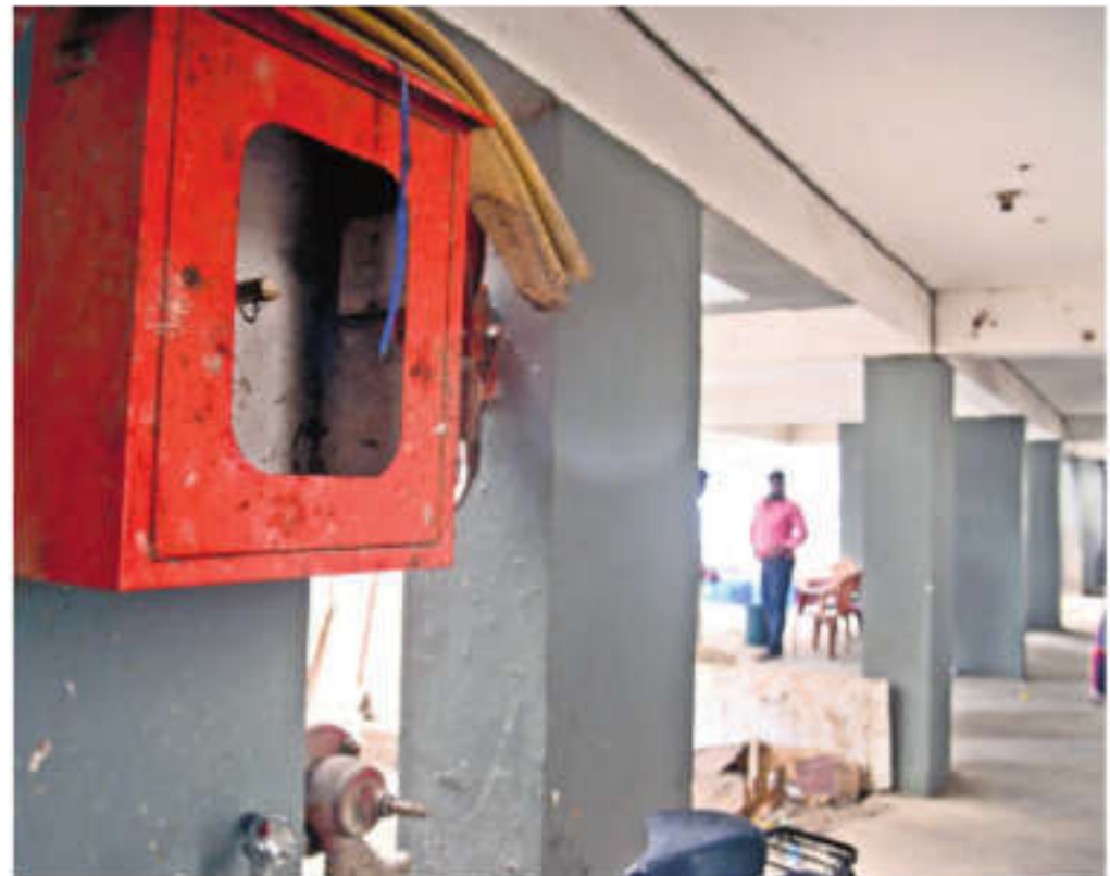
Empty fire extinguisher boxes and narrow, broken staircases at TNUHDB tenement in KP Park, Pulianthope, pose serious risk in case of fire accidents | MARTIN LOUIS
